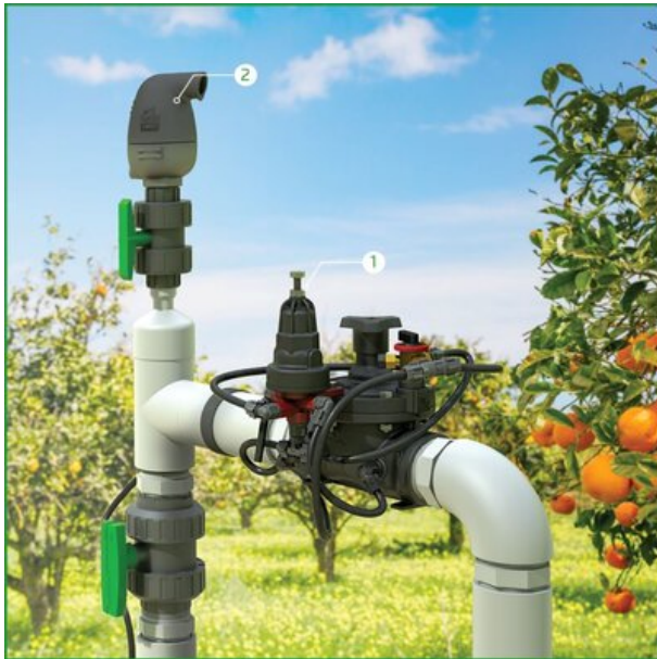
[1] BERMAD Model IR-220-50-3W-XZ Opens upon pressure drop, and establishes reduced pressure zone protecting laterals and distribution line.
