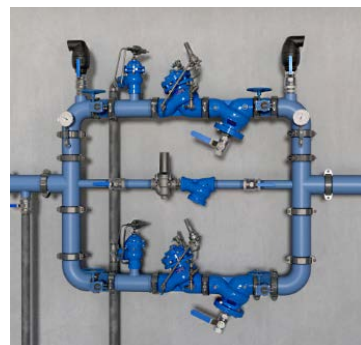
Picture 4.8 – On Floor pressure reducing station
