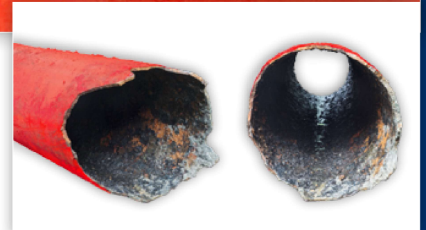
2. Piping breached by water hammer
