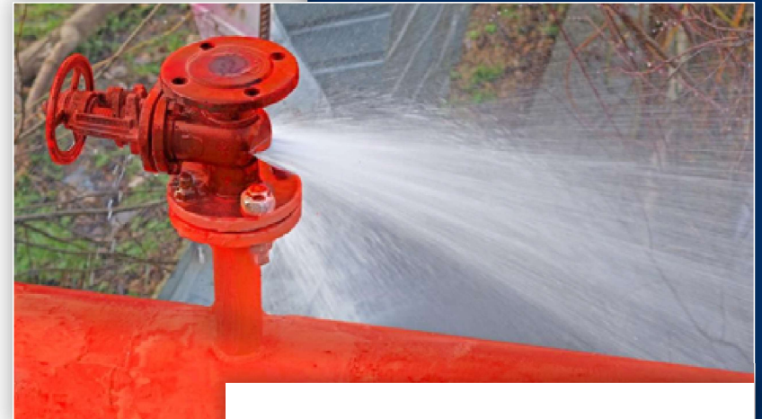
1. A valve casing cracked by surge pressure
