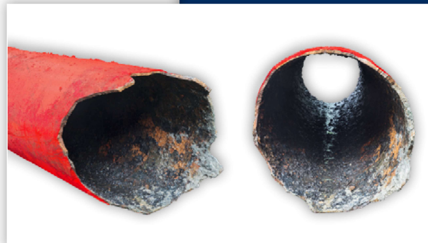
2. Piping breached by water hammer
